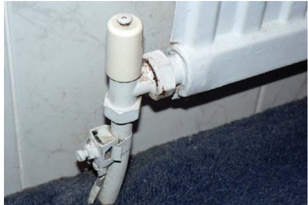
Unmarked bonding conductor
