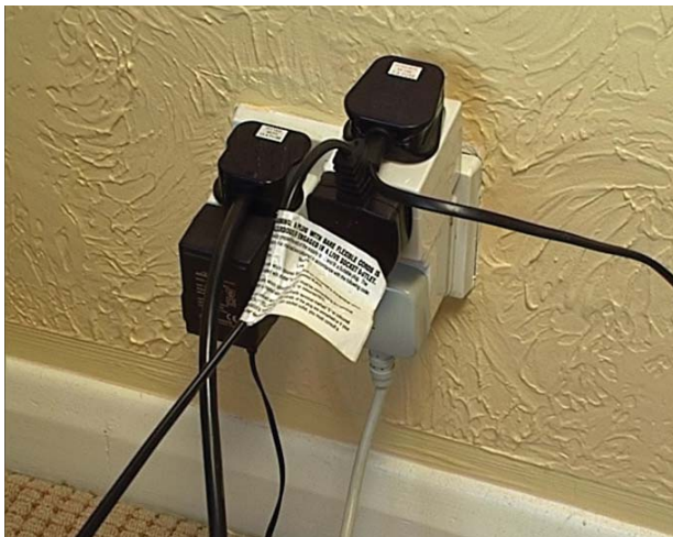
Potentially overloaded socket-outlet
