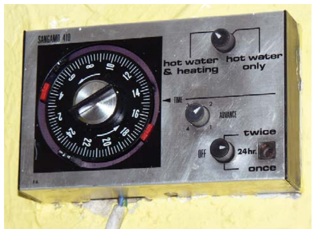
Cable sheath not taken inside enclosure
