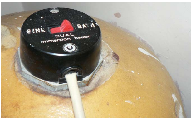
Older immersion heater without thermal cut-out
