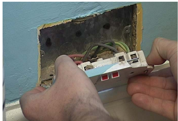
Socket-outlet with broken face plate
