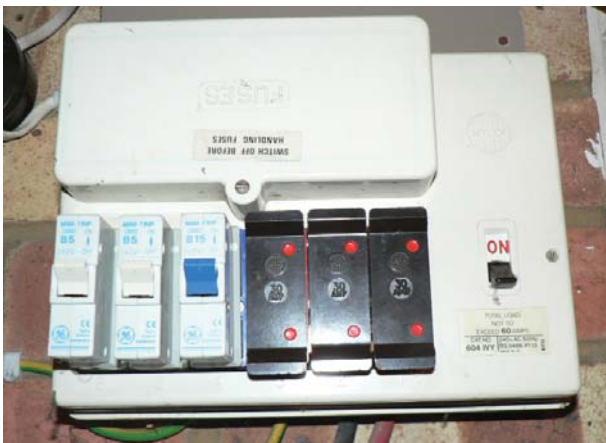
Consumer unit with fuses and circuit-breakers
