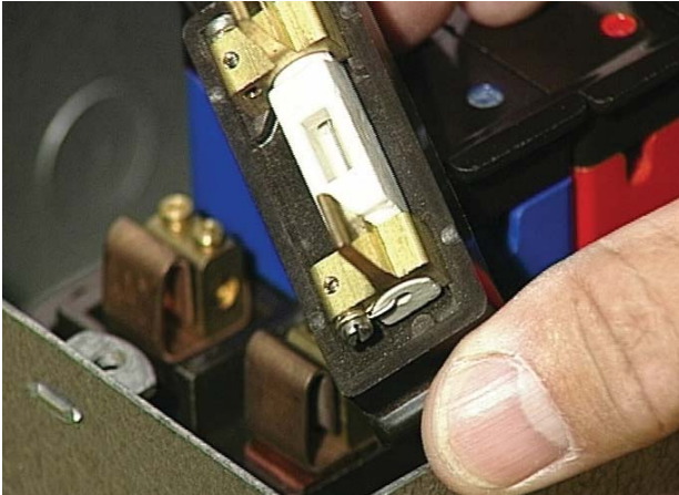
Checking a fuse carrier
