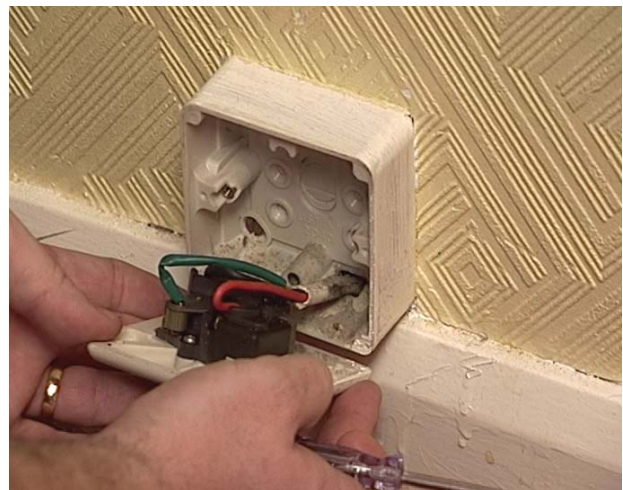
Inspecting a socket-outlet
